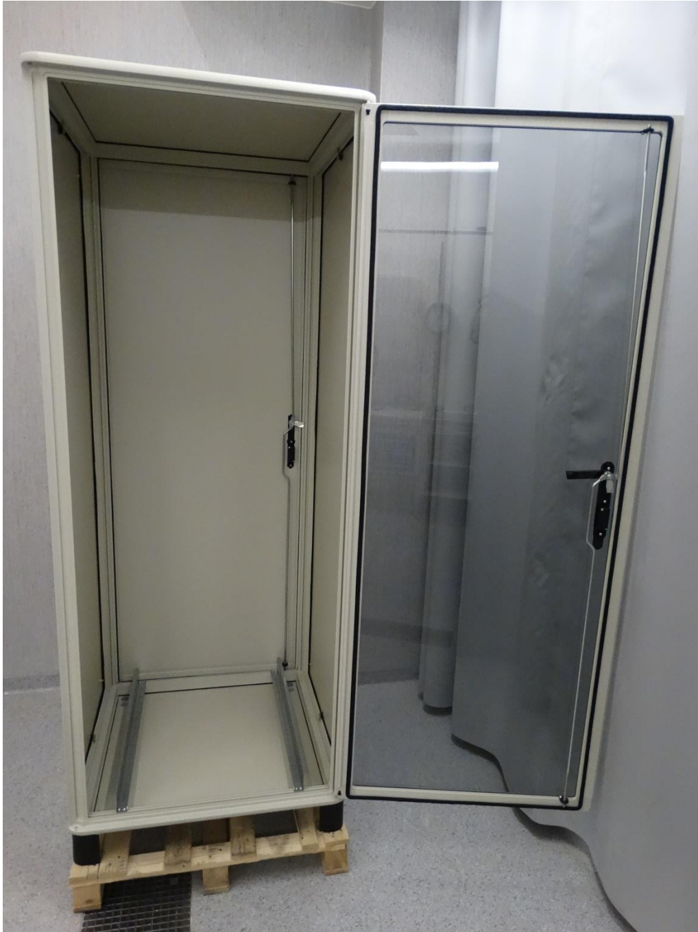
Photograph 5: Fs1 cabinet, door opened
